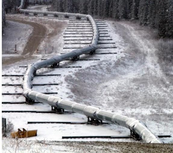
Ruptured oil pipeline
